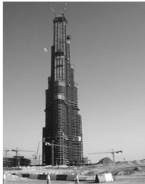
Under construction: the Burj Dubai, the world's tallest building. The actual height is a closely guarded secret and won't be revealed until construction is completed.
